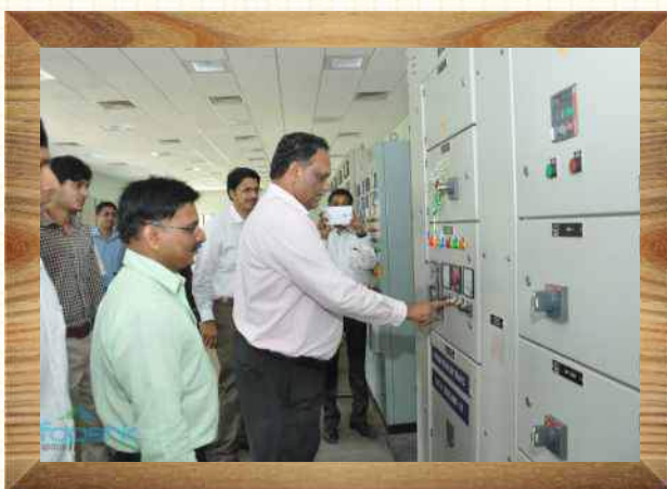
Switching on of 110 KV substation at cherthala
